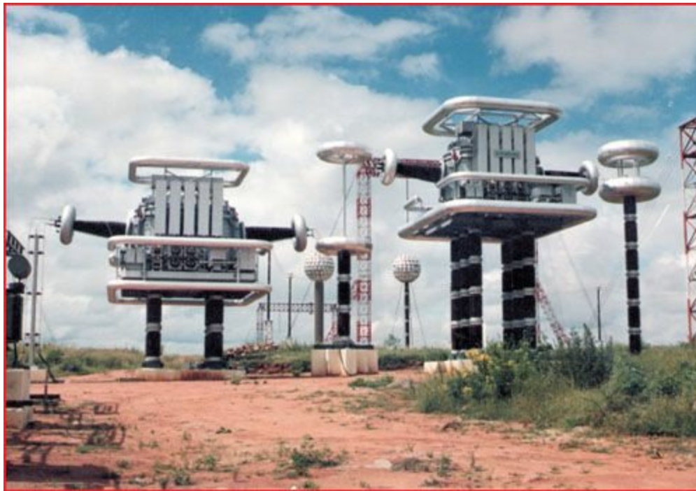
1600 Kv, 9600 kVA Outdoor Type Cascaded Power Transformers. Courtesy: Central Power Research Institute, UHV Lab. Hyderabad, India.
