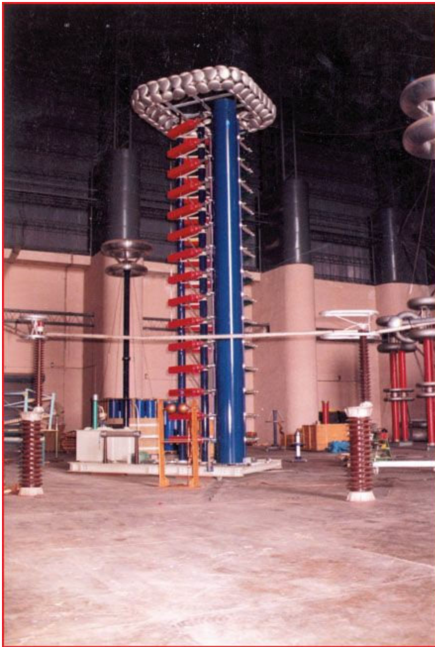
3 MV, 150 KJ, 15 Stages Impulse Voltage Cenerator. Courtesy: Central Power Research Institute, Bangalore, India.
