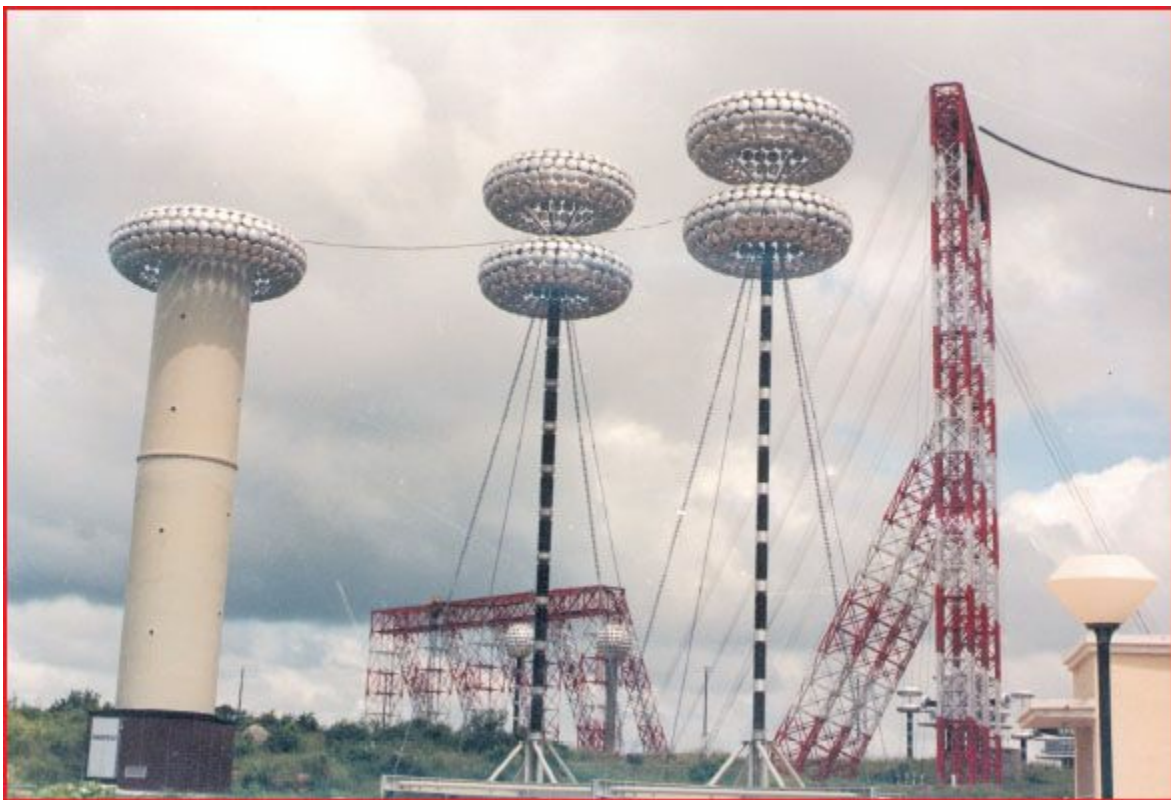
5 MV, 500 KJ Outdoor Type Impulse Generator with Damped Capacitive Divider (600 pF, 400 Ohms), and Loading Capacitor (2 nF) both rated for 4.4 MV Lightning Impulse and 3.7 MV Switching Impulse. In the picture Impulse Voltage Generator is shown on the left followed by the load capacitor and the damped capacitive divider. Courtesy: Central Power Research Institute, UHV
